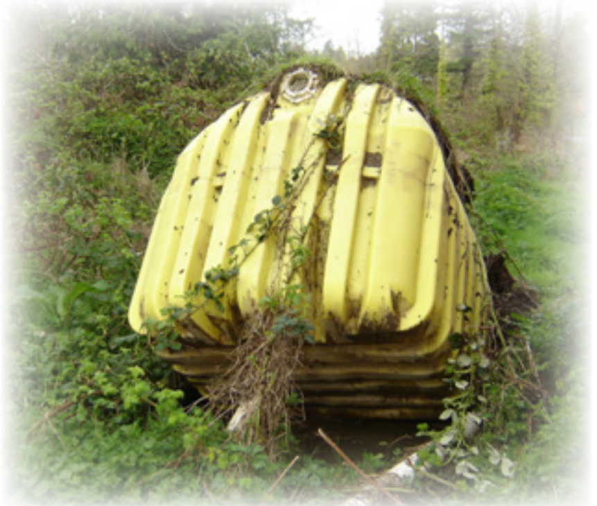
Pierce County: Empty poly tank surfaces due to a high water table.
